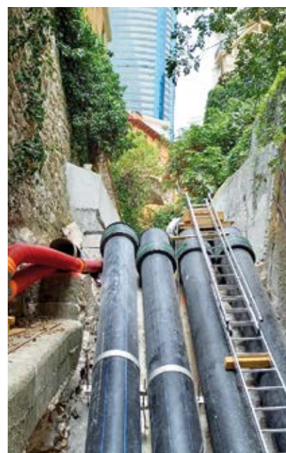
The PE pipeline for the further transport of the heating/cooling energy
